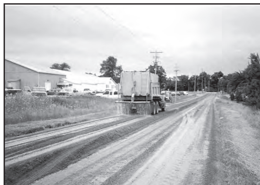
c) Shaping the stabilized material and adding water to optimum moisture condition for compaction.
