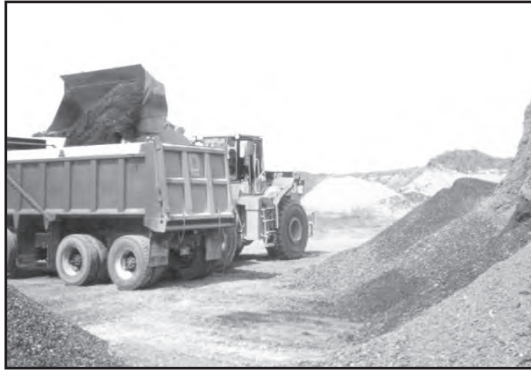
a) Loading of stockpiled cold recycled asphalt into dump truck for paving
