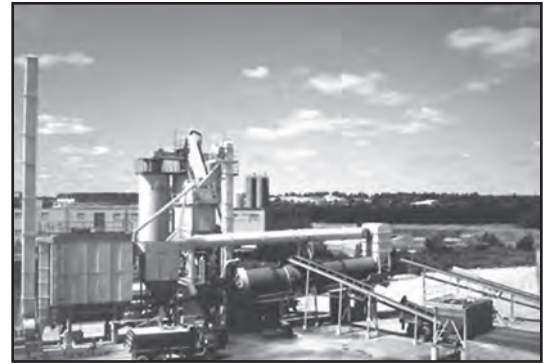
Photo 3-2: Typical counterflow drum-batch asphalt plant
