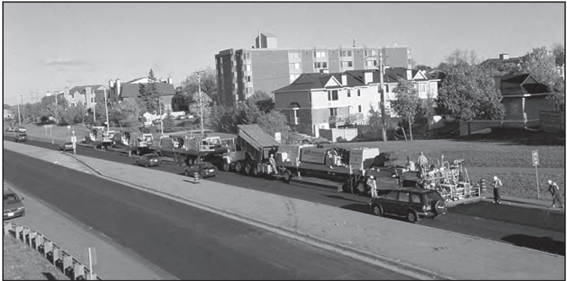
Photo 3-3: Current HIR Remixing train rehabilitating a municipal roadway in a single pass, 2002
