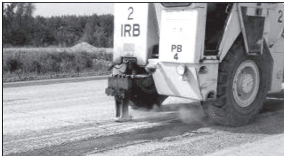
Photo 3-10: A resonant breaker in operation in Oxford County, Ontario
