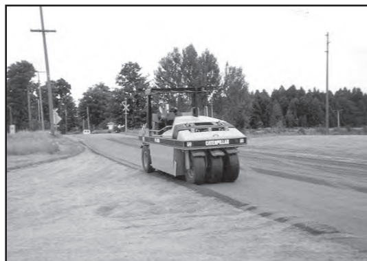
d) Initial compaction with heavy rubber tired roller followed by vibratory steel roller.
