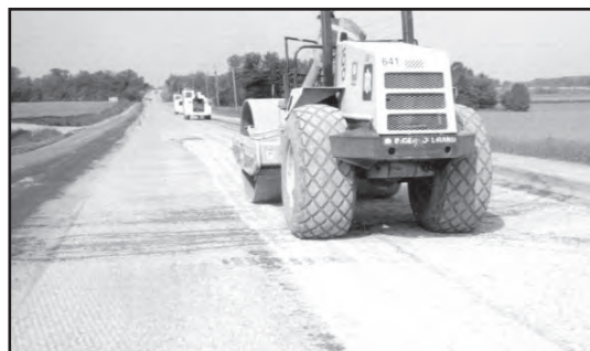
c) Low amplitude compaction of the rubblized PCC using a steel drum roller.
