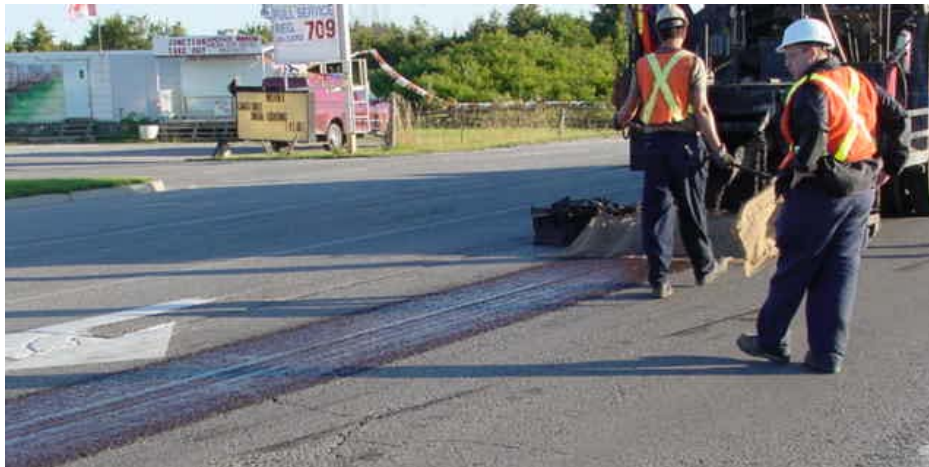
Figure 3–8: Pre-treating of moderate alligator cracking at the centerline with a strip of micro-surfacing prior to applying a regular course of micro-surfacing on the entire surface. (Courtesy of Ontario Ministry of Transportation.)
