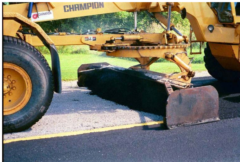
Figure 3–2: Application of a scratch coat of a densely-graded hot mix by a grader with box-like attachment. (Courtesy of Ontario Ministry of Transportation)
